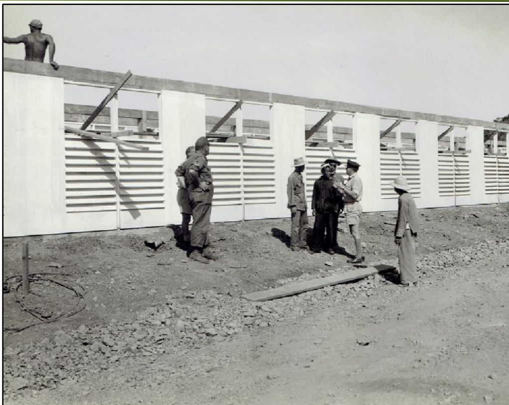
The Red Horse Top Sergeant (left) with the RAAF interpreter (right) instructing local civilian employees at the RAAF Quarters, under construction.
