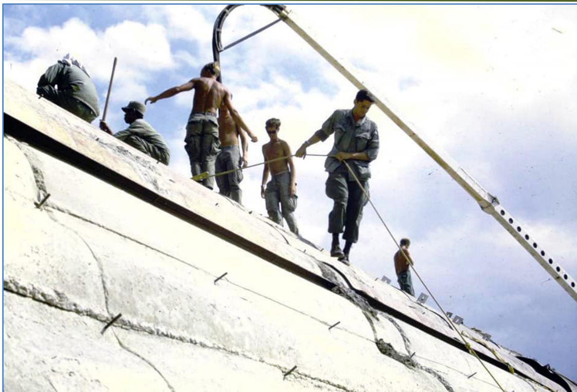
Concrete being poured on the structure. Construction occurred in the fall of 1969. The concrete had to be pumped to the top of the structure via a special concrete pump.
